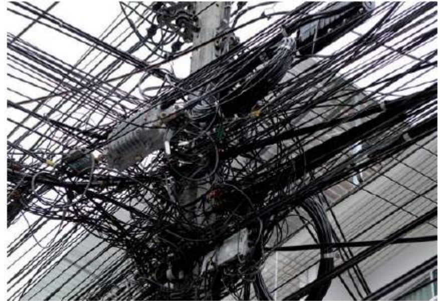
■ Figure 10.21 Power line spaghetti
