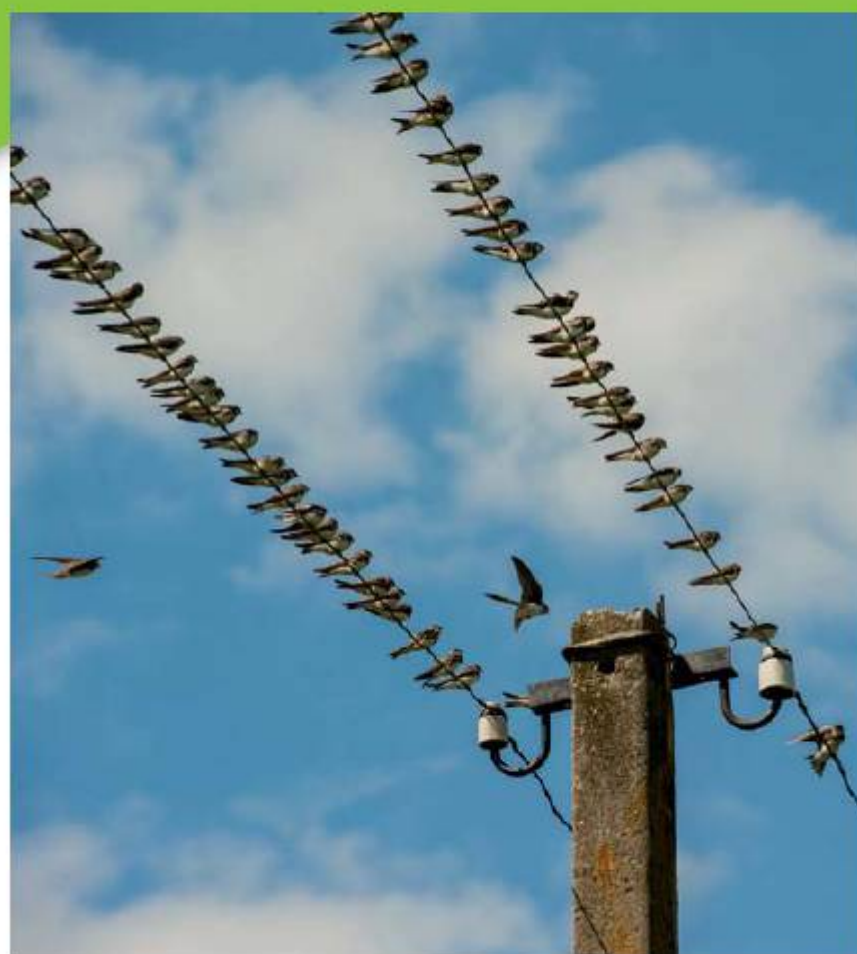
■ Figure 9.28 Birds can sit unperturbed on high-voltage cables
